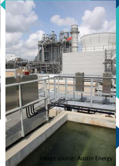
Wastewater effluent cooling a combined cycle power plant
